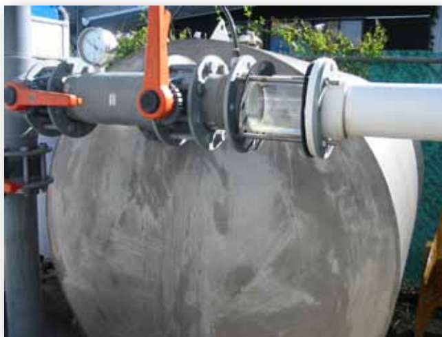
The clear poly pipe is the sight glass for the backwash water, which will show the water reducing in turbidity as the backwash cycle is completed.
