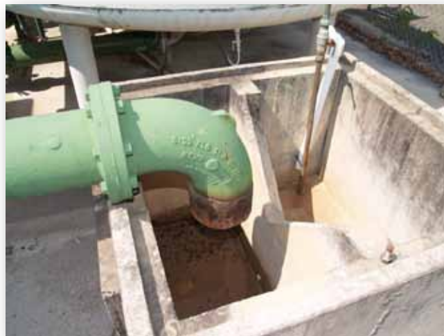
All open drains should be covered.
