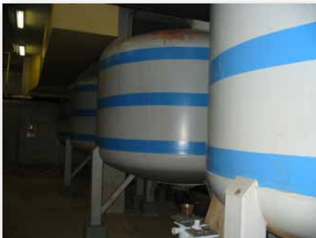
Steel sand filters.
