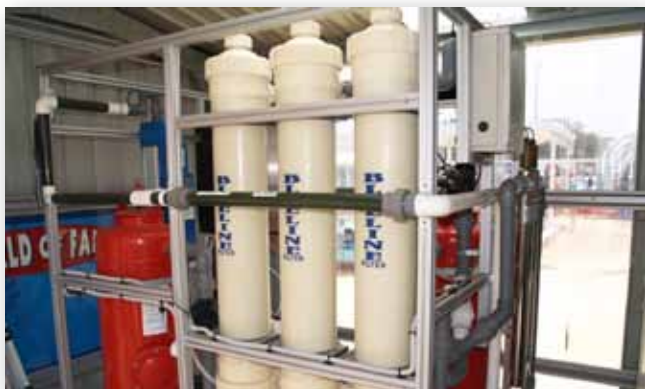
A backwash water recycle unit.
