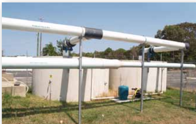
A water recycling plant.
