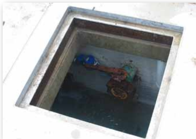
An open balance tank poses enormous risk to the staff of an aquatic centre and the patrons.
