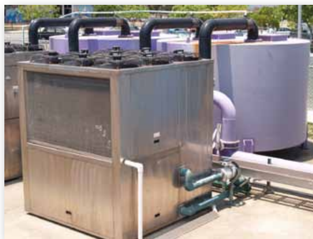
Electric heat pumps are common in large complexes.
