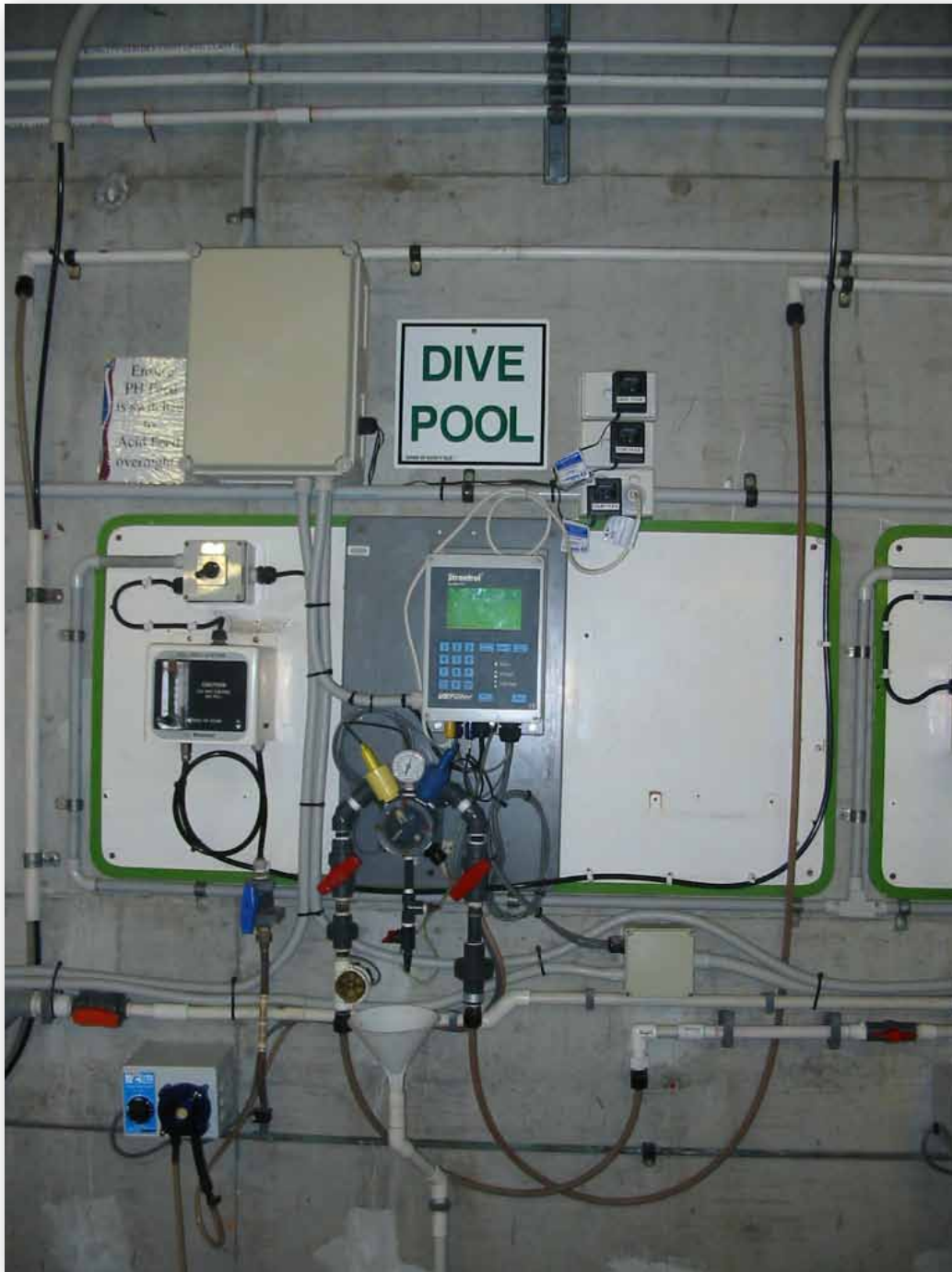
An automatic dosing unit used to inject chlorine into the pool water system
