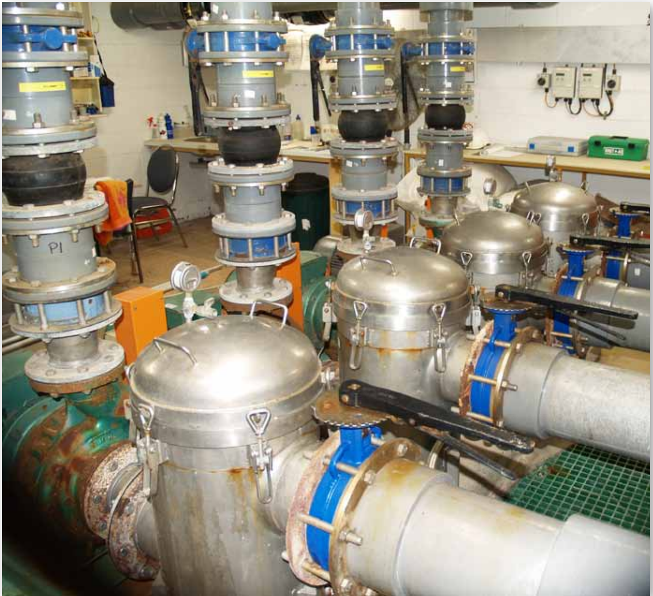
A large plant room with inlet pipes leading to lint baskets and water is then pumped under pressure to the filters.
