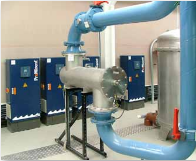
UV Treatment System
