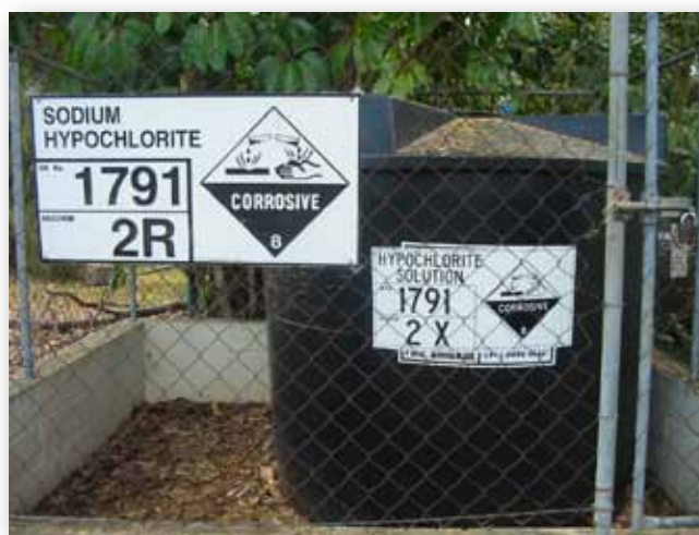
A chlorine storage tank
