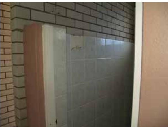
Broken tiles in change room.
