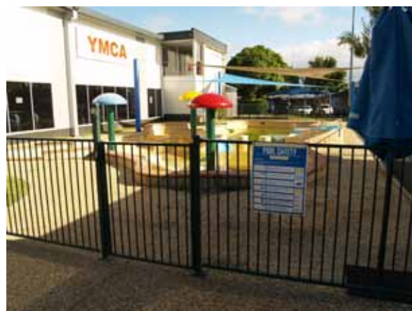
Wading pool fence in need of repairs.
