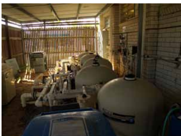
Plant room to be cleaned up.
