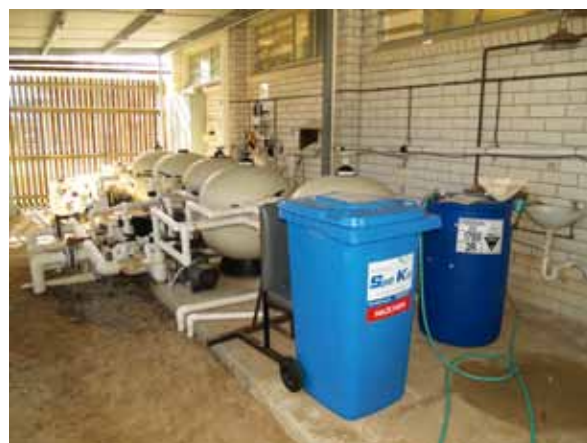
Tidy plant room.
